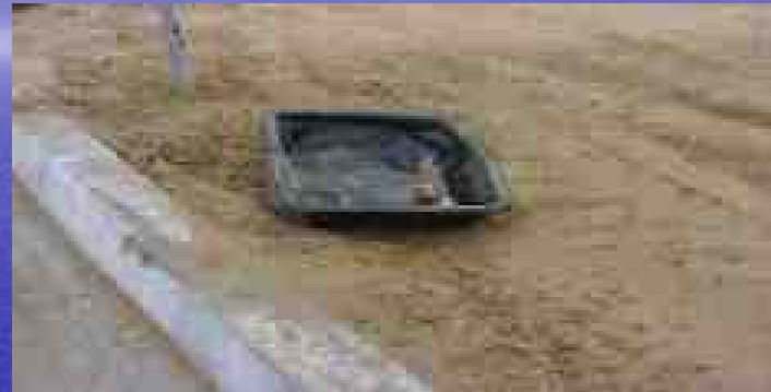
Damaged drip pans
