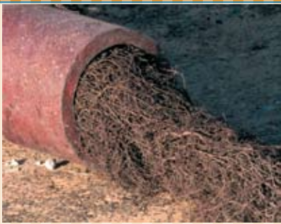
▲ © Root-Damaged Lateral Pipe by John Miner
