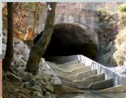
Friends of Corte Madera Creek Watershed used grant funds to install the Lansdale Station fish ladder. Now, fish can migrate upstream.
