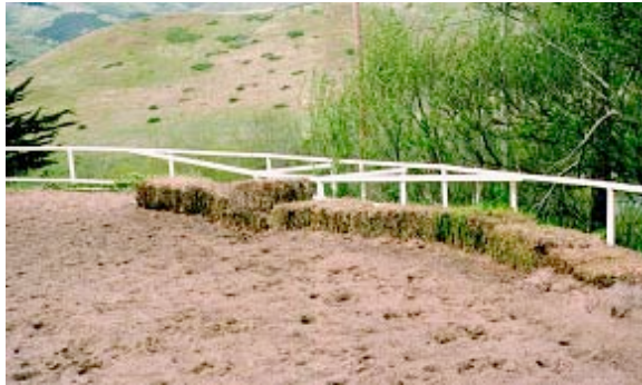
A straw bale sediment barrier retains sediment while allowing water to pass through. Bales need to be anchored with stakes or rebar. Be sure that water cannot flow around the barrier and cause downslope erosion.
