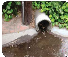
Residential runoff that drains to the street contributes to localized flooding.
