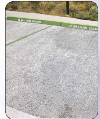
Pervious concrete is used in parking areas at The Marine Mammal Center, Sausalito.
