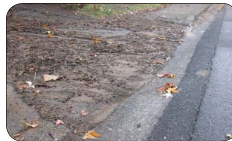
AFTER A RAINSTORM, SEDIMENT RUNS OFF A ROAD AND INTO A GUTTER. SEDIMENT IS THE NUMBER ONE POLLUTANT IN MARIN CREEKS!
