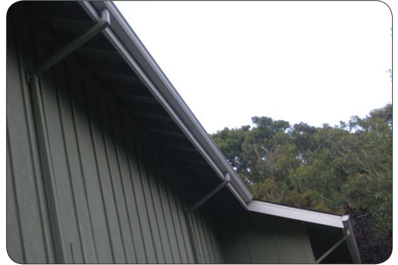
Adding additional downspouts helps reduce the volume and velocity of runoff at any given point. This, in turn, reduces the potential for erosion as it comes out the downspout.
