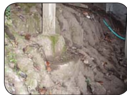
Visible erosion under a deck is common.
