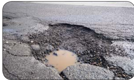
"POTHOLE" CAUSED BY...
